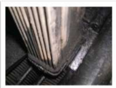
Oil washed base of Cooler
